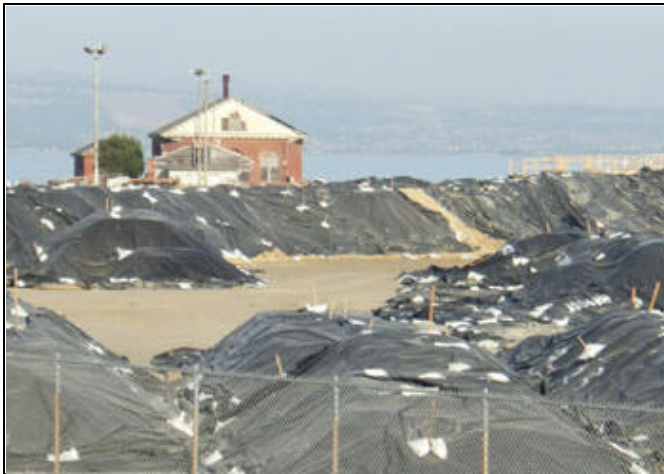
At the former naval shipyard at Hunters Point, cleanup efforts this year involved excavating 25,000 cubic yards of pipes and soil that had to be scanned for radiological residues. Photo by Arthur O'Donnell.
